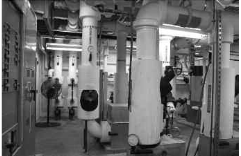
GEOTHERMAL HVAC SYSTEM AT HIGHLAND ELEMENTARY SCHOOL
